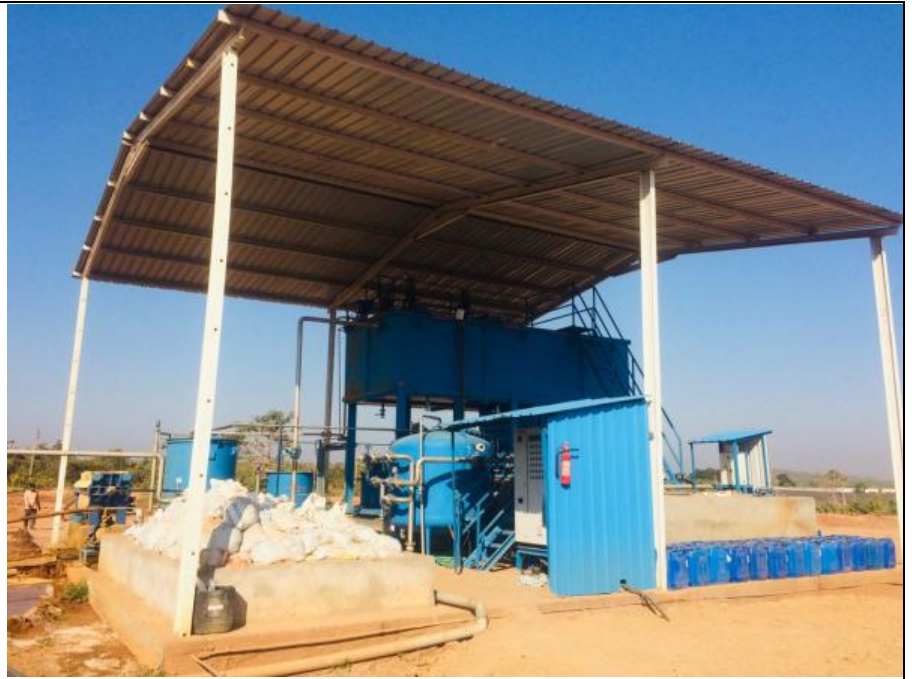
Primary Effluent Treatment
