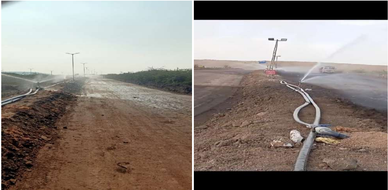
Fixed type water sprinkling system provided to check dust emissions at project
